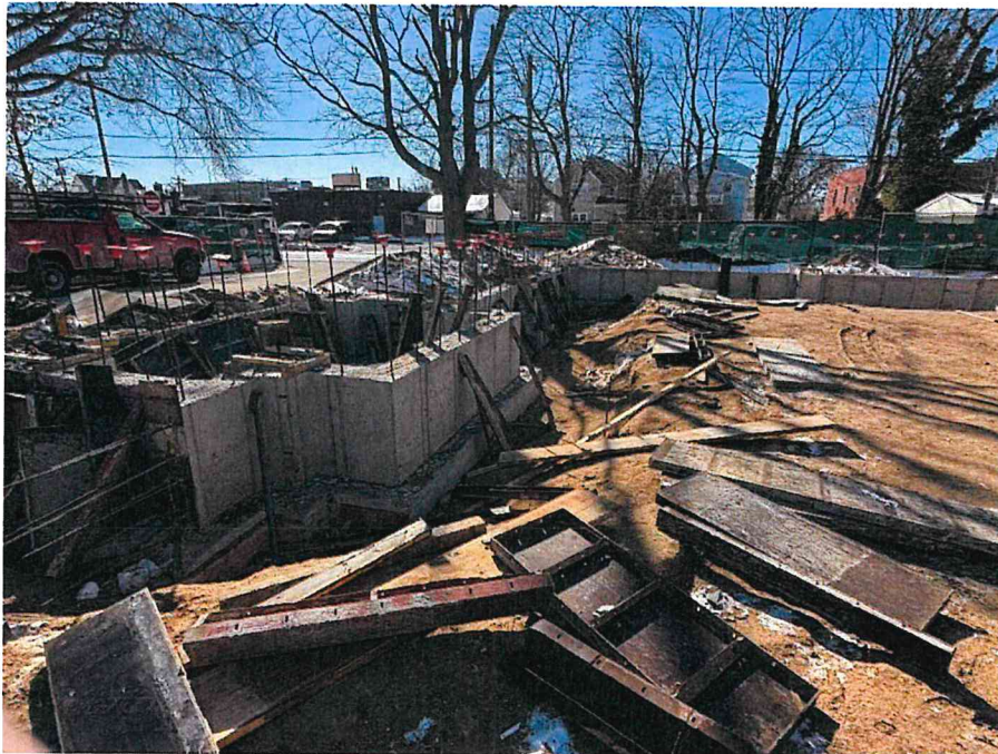
Stalco, concrete subcontractor York pouring and then stripping the new foundation walls.
