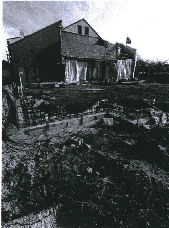
Stalco concrete subcontractor York Pouring the new addition footings on the north and south side of the new building.
